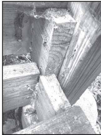
This shows small little screws unattached and no braces, causing the Cupid Falls elevated walkway to collapse.
